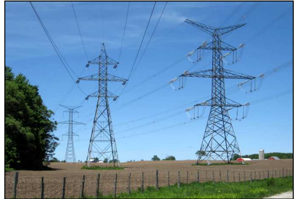
After 230kV + New 500 kV Transmission Lines
